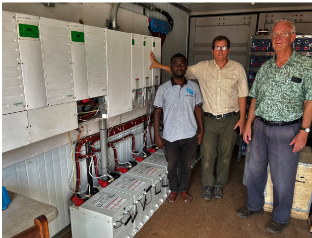
This 17 KVA system will be expanded to 51 KVA.
